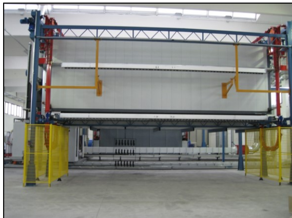
Curing oven exit door
