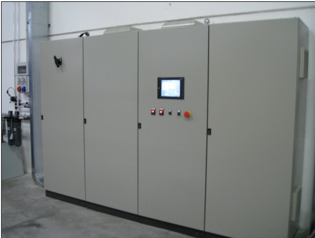
Main electric board
