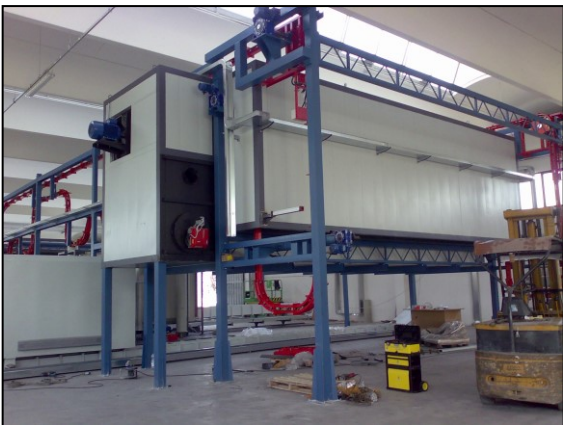
Curing oven zone
