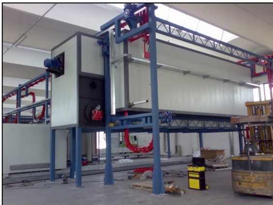
Curing oven zone
