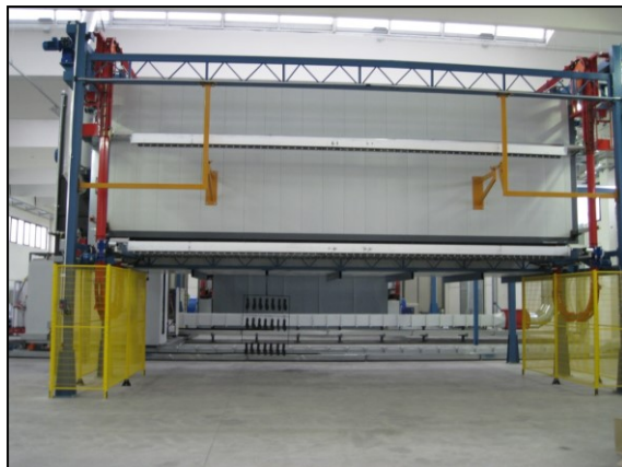
Curing oven exit door
