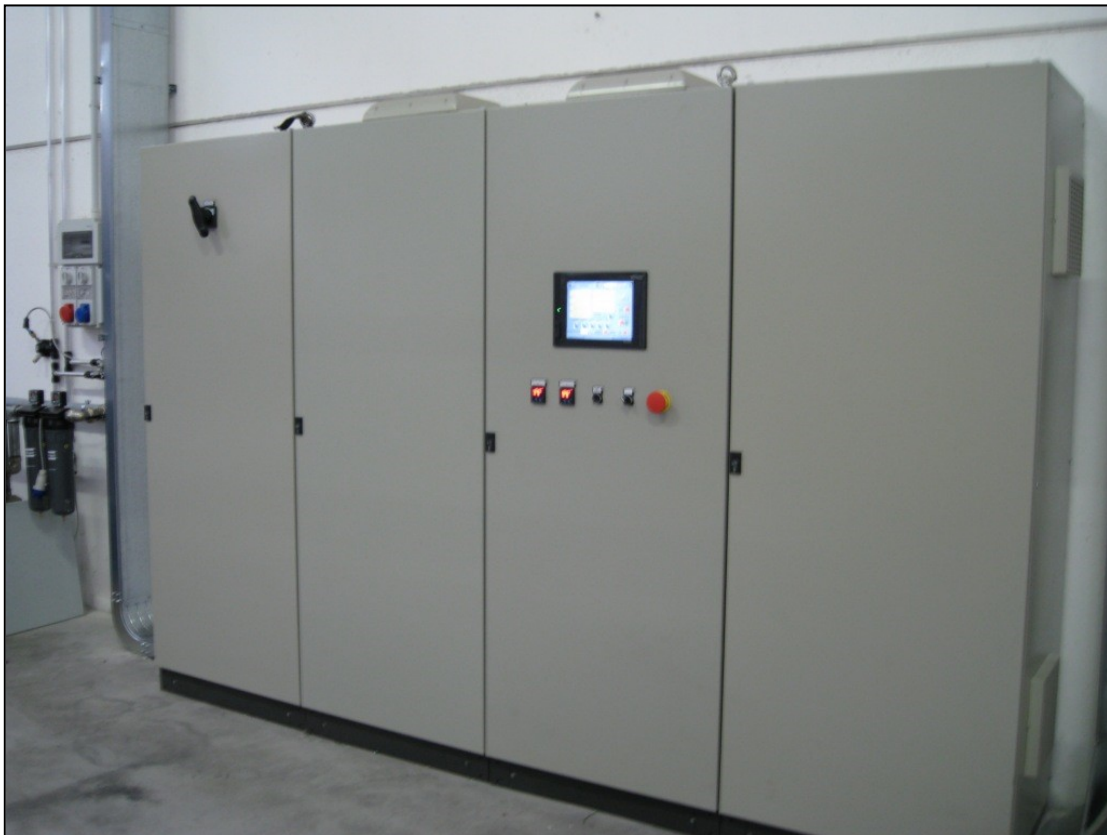
Main electric board
